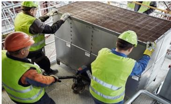
Installation stationary DNOx catalyst
